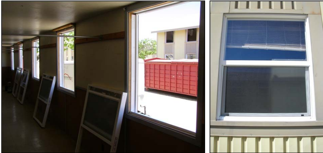
New energy efficient windows were installed in place of the old windows.
