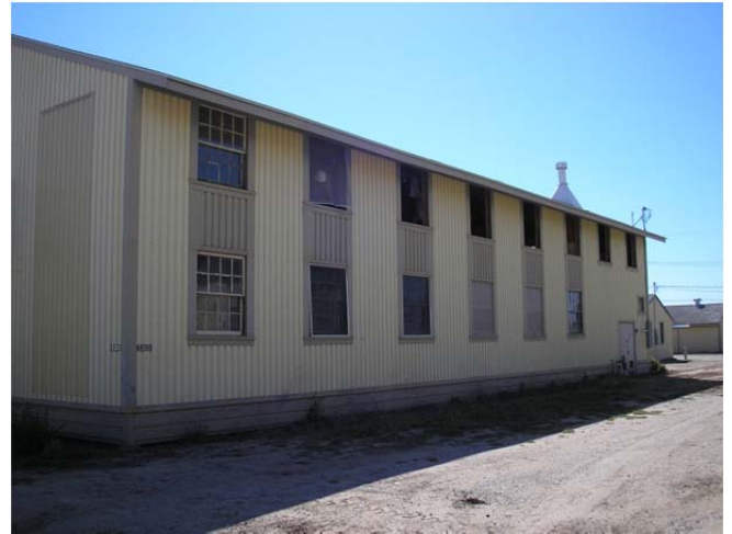
Above is one of the many buildings that required the windows to be replaced.
