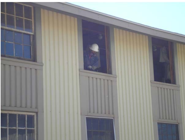
The windows were removed and disposed of LBP by the abatement subcontractor.
