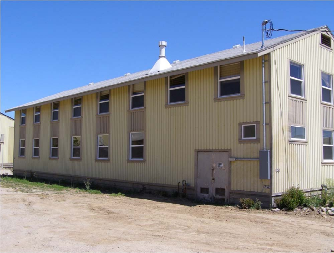
The rear-view of a building shows one of the 170 new subpanels which were also installed as part of this project.
